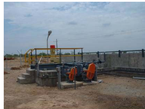
4. Limestone slurry tank, feed and recycle pumps
