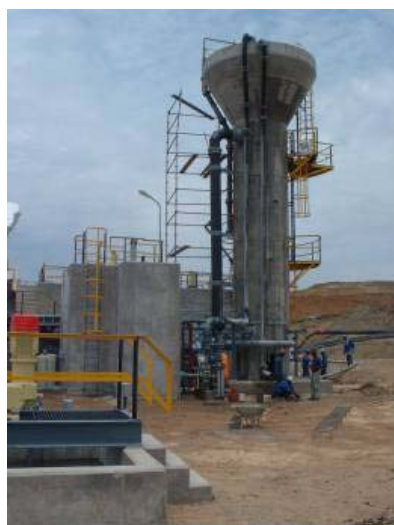
5. Iron(II)-oxidation and Fluidised-bed reactors
